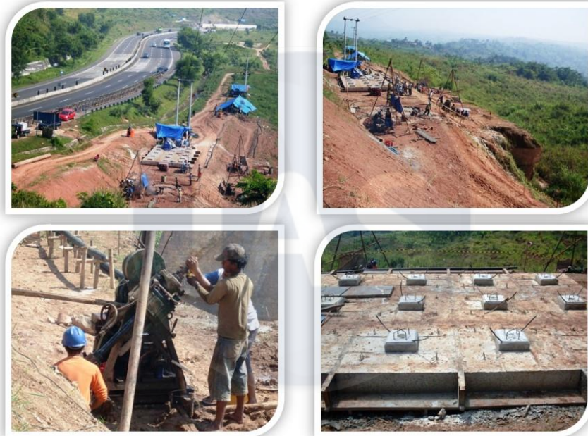
Anchors as one of internal slope reinforcement at Cipularang tol road
