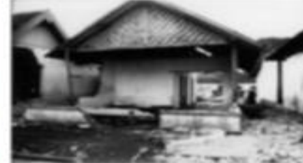
Figure 10. Typical damage to a beach house located about 100 m from the sea at Banyuwangi.
