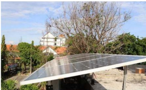
Picture 7 Solar Panel at Engineering Physics
