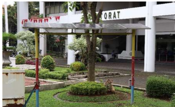
Picture 6 Solar Panel at Rectorat Building
