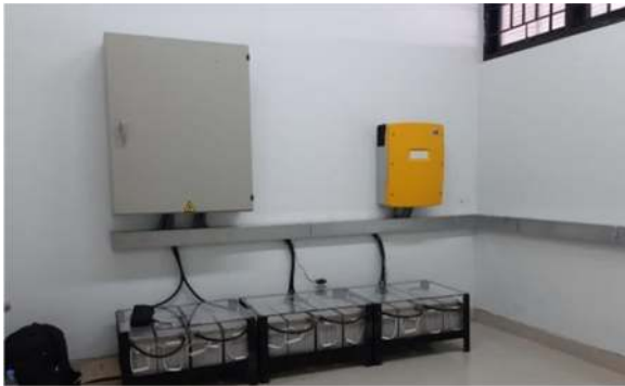
Picture 3 Solar Panel's Battery at Electrical Engineering
