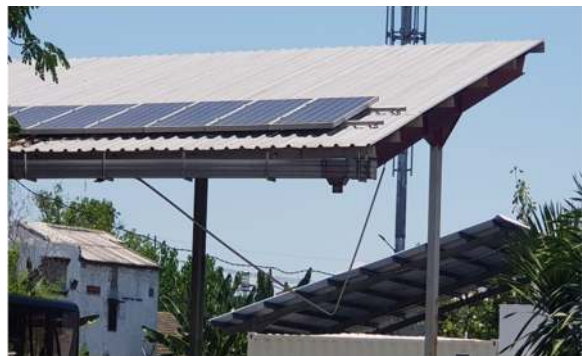
Picture 8 Solar Panel at Robotics Building
