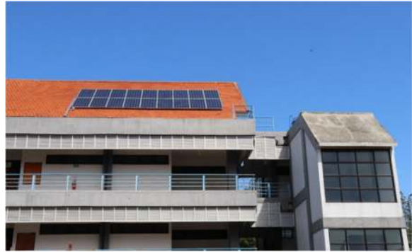
Picture 2 Solar Panel at Electrical Engineering
