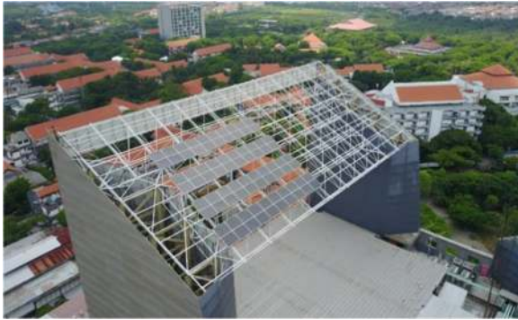
Picture 1 Solar Panel at Research Center Building
